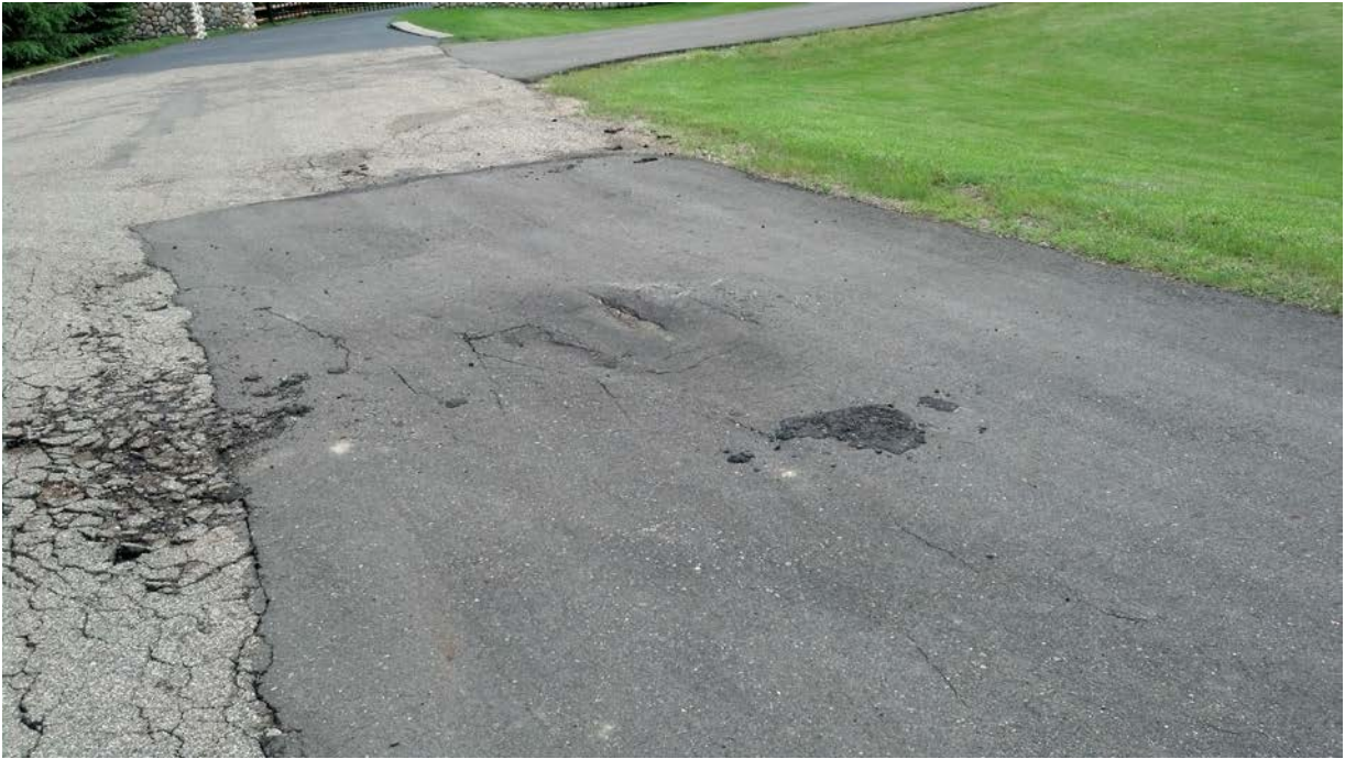
Figure 13: Picture to show failure modes of Schurman Drive-Picture by Francis O. Dayamba
