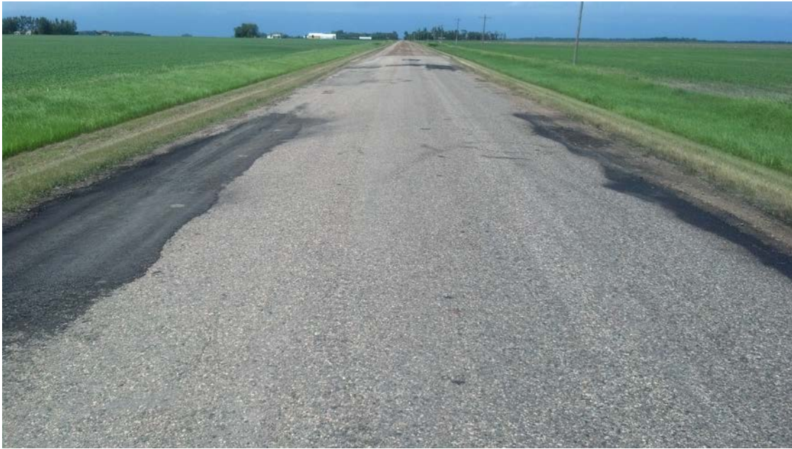
Figure 14: Picture to show failures of CO 95-Picture by Francis O. Dayamba
